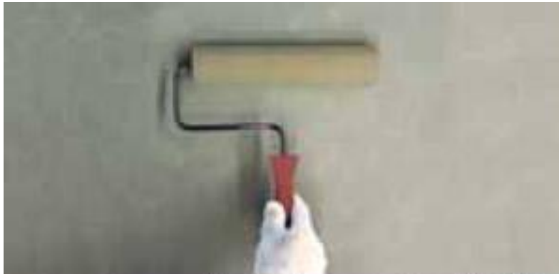
Sealing of a self smoothing floor with a mat sealer, using a short pile roller
