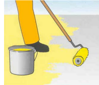
Even application of Primer coat Sikafloor®-156 and the conductive Layer Sikafloor®-220 W Conductive : with medium to long haired roller or brush. E.g. Polyplan roller and brush.
