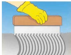
Spreading of Sikafloor®-235 ESD with notched trowel. E.g. Polyplan notched trowel 5/7 mm.
